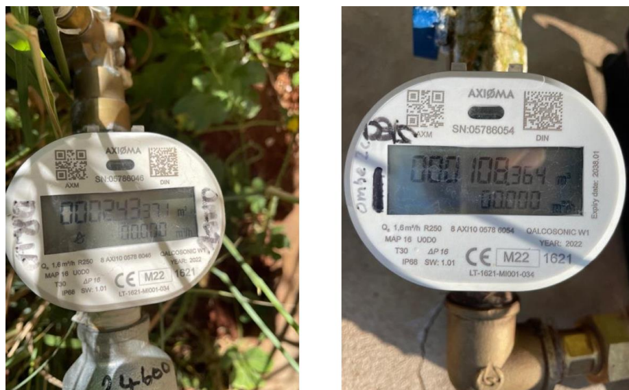
Figure 2. Axioma flow meters in SLECI and surface drip irrigation
